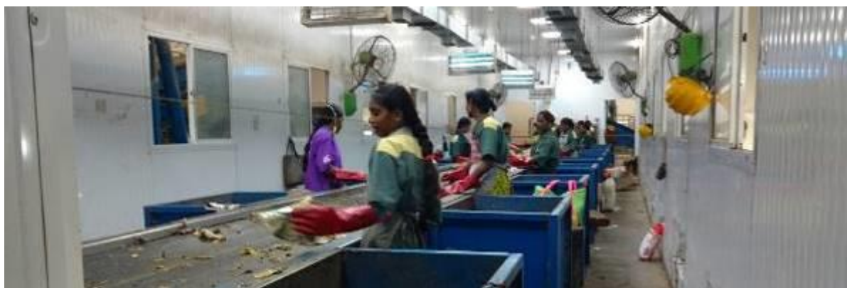
Image 9 Solid waste treatment facility at Salegaon (segregation Belt)
